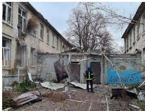
Damaged kindergarten in the city of Severodonetsk, Luhansk region
